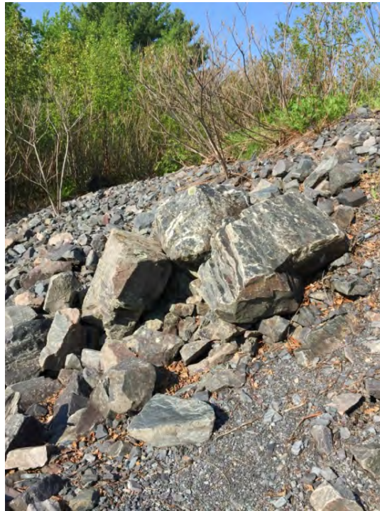
Photo No. 3 – View looking southwest of the downstream slope of the right embankment. Note the heavy riprap and small vegetation.
