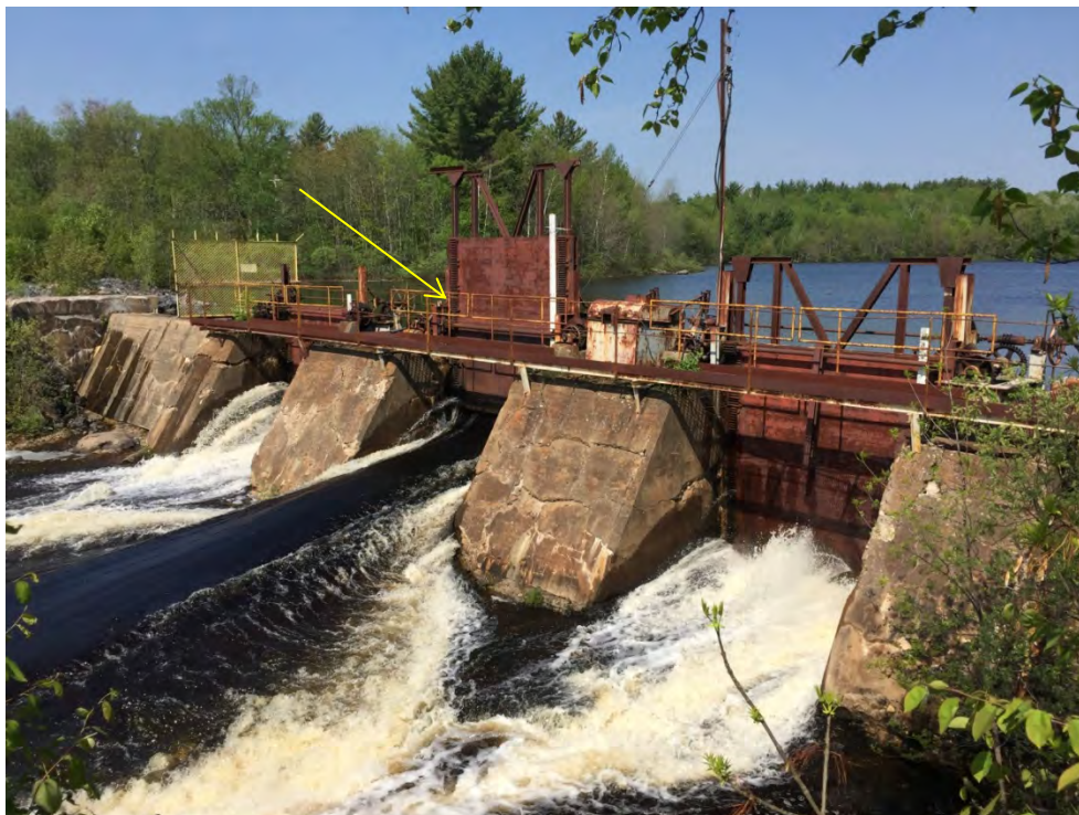
Photo No. 2 – View of the downstream side of the dam looking west. Note the open middle slide gate.
