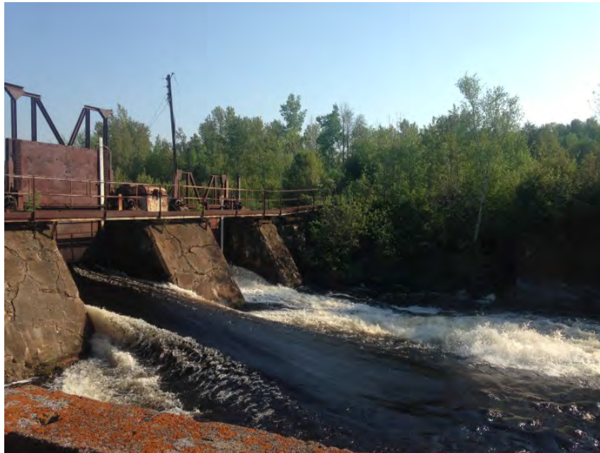
Photo No. 5 – View looking north, showing the downstream face of the dam and the heavily vegetated left embankment.
